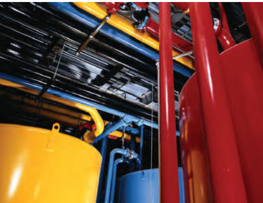
Compressed Air Systems
